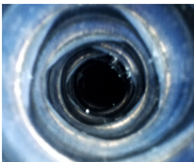
5. Damaged channel at bending section (compressed)
