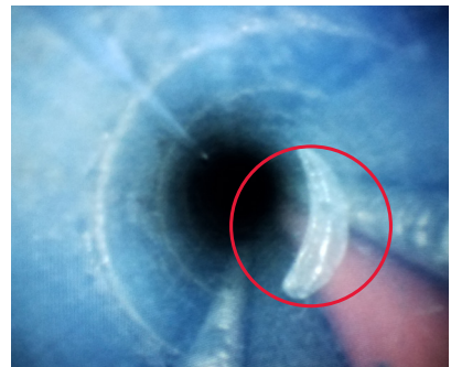
3. Cut or tear in channel
